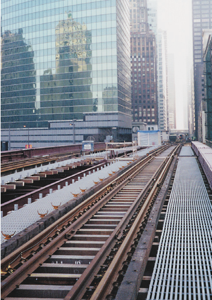
Chicago Transit maintenance walkways alongside elevated train tracks constitute one of the largest fiberglass grating installations in history. This project used T-5000 2" with a custom polyester resin.
