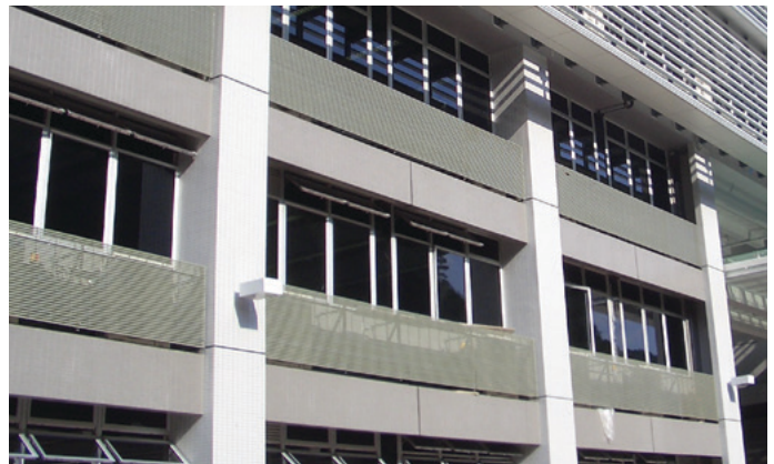
Strongwell I-6000 grating was installed at this School of Business and Information Systems in Hong Kong as air-conditioning platforms when placed horizontally and as louver when placed vertically (as shown here).
