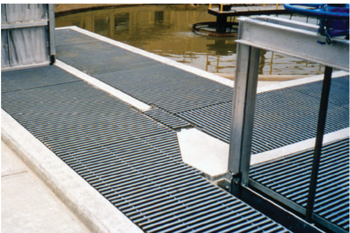
Low maintenance fiberglass grating provides trouble free operations for the covers and walkways in the Lakewood, Colorado Wastewater Treatment Plant Headworks. I-6000 1-1/2" was used.
